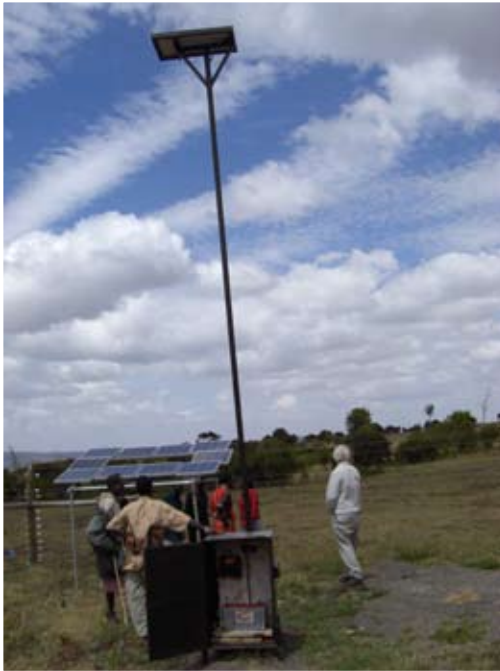
Solar panels and bore hole
